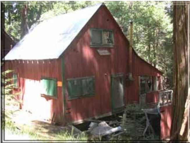
Figure 30: The County has condemned this house as seen by the orange notice posted on the siding. Half of the porch has collapsed leaving a pile of wood susceptible to ignition. Photograph by Timothy Walsh.
