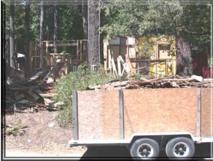
Figure 27: This home is being remodeled and has piles of construction debris covering the parcel. Residents stated that this parcel has been in this condition for some time. Photograph by Timothy Walsh.
