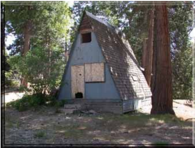
Figure 42: The small A-frame shack next to the old lodge needs to be razed. In its current condition, embers will blow in through the openings in the plywood or vent hole. Once ignited, burning wood shingles will travel several hundred feet threatening several neighboring structures. Photo by Timothy Walsh.
