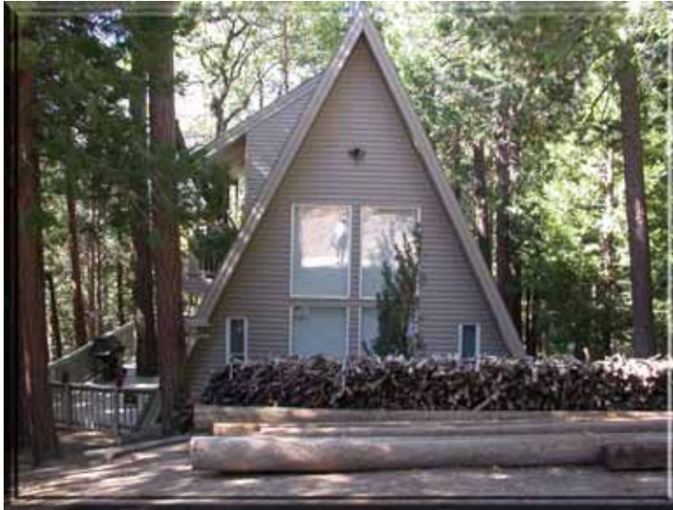
Figure 25: This house has firewood stacked in several places. The small diameter of the wood will readily ignite and the heat output could exceed the protection offered by the metal siding. Photograph by Timothy Walsh.
