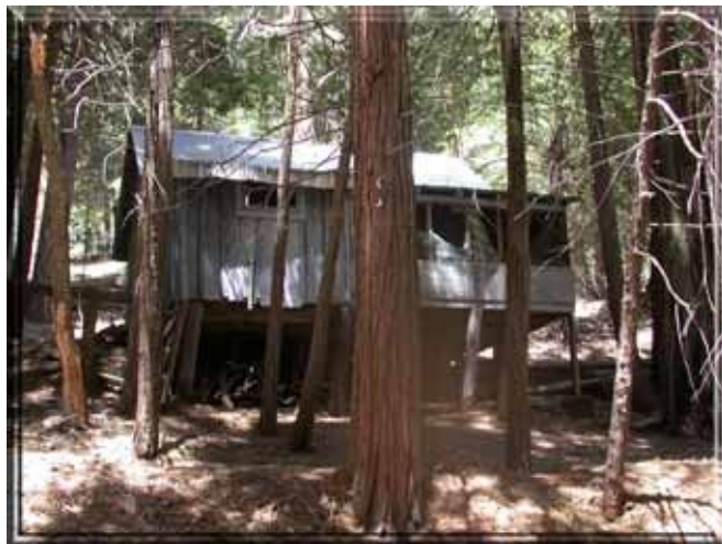
Figure 48: 8501 Old State Road appears to be falling off the support timbers. Photo by Timothy Walsh.
