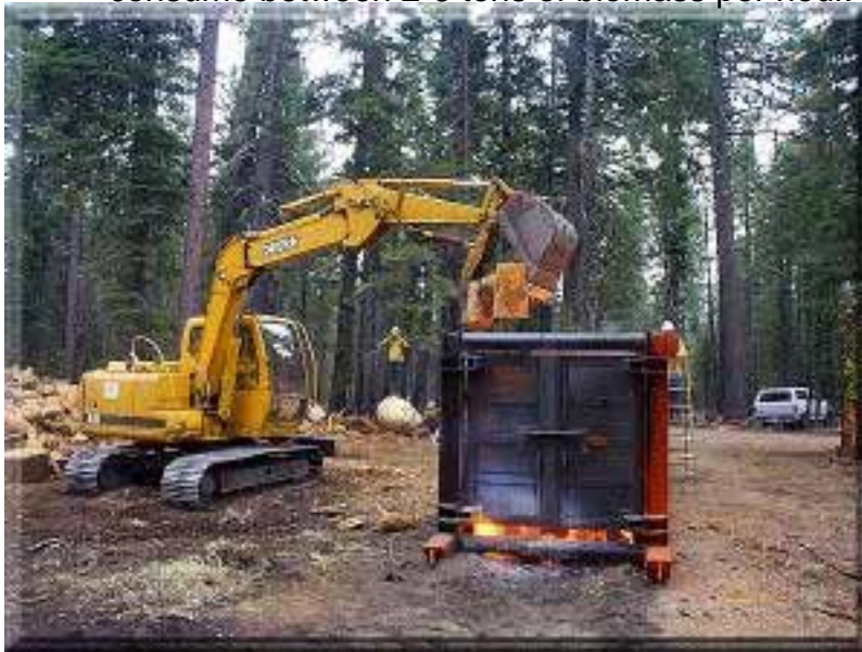
Figure 75: An air curtain destructor in use in Lake Tahoe reducing debris from bug infested trees. Photo from the Airburner website.
