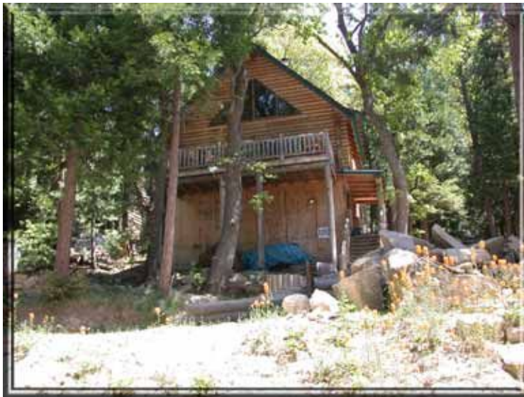
Figure 26: This house has a tarp covering firewood next to 1/2 or 5/8 inch plywood found under the deck. This tarp would ignite easily and burn with high enough intensity to ignite the plywood. Photograph by Timothy Walsh.
