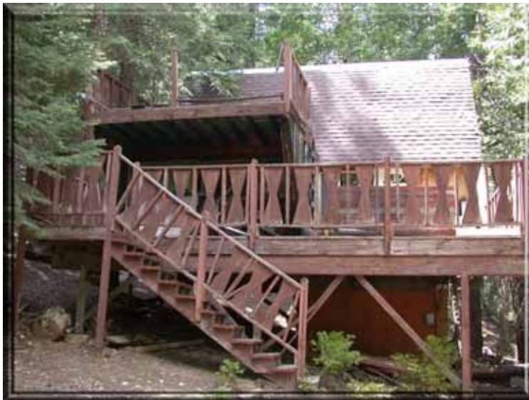
Figure 28: Boards stored under the deck could easily ignite during a wildland fire. Photograph by Timothy Walsh.
