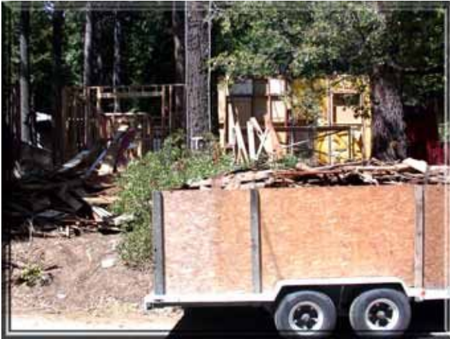
Figure 49: The home located at 8817 Old State Road with the construction debris left on site. Photo by Timothy Walsh.
