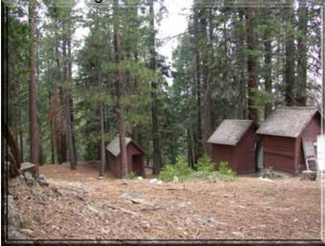
Figure 83: An example of the buildings found at Camp Kaweah. Notice the wood shake roofs. The shack in the middle has a hole in the roof.
