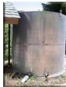
Figure 92: A 4000-gallon water tank.
