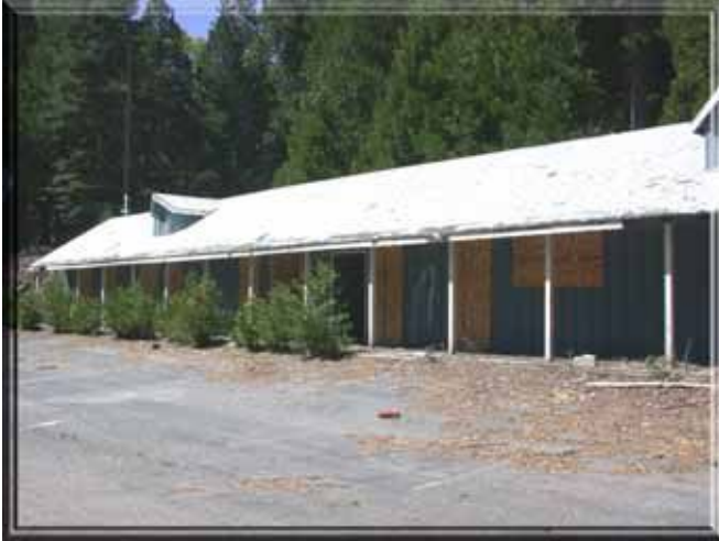
Figure 41: Small trees and piles of forest debris are under the eaves of the old lodge. During a wildfire, these combustibles may ignite the abandoned building. Photo by Timothy Walsh.
